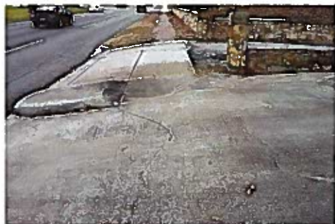
Non-compliant cross slope
