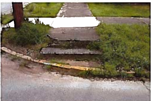
Missing ramp - steps
