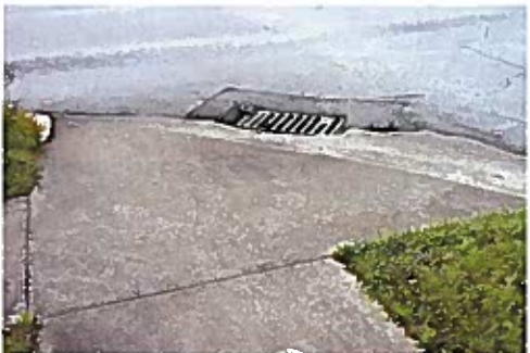
Storm drain blocking ramp
