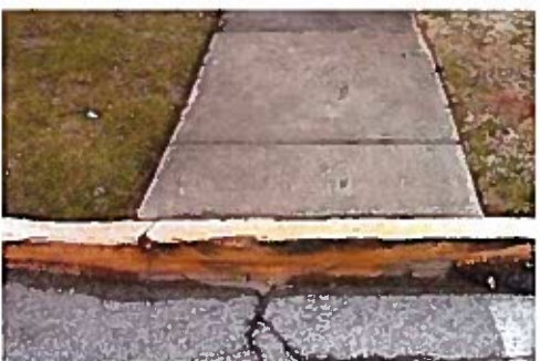
Missing ramp - curb
